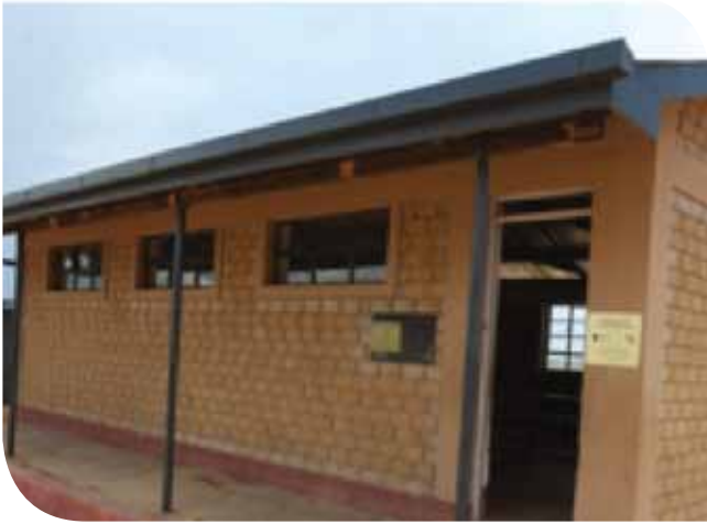
A new classroom at Mwaluvuno Primary school donated by Safaricom Foundation through the Know and Grow Education Programme Partnership
