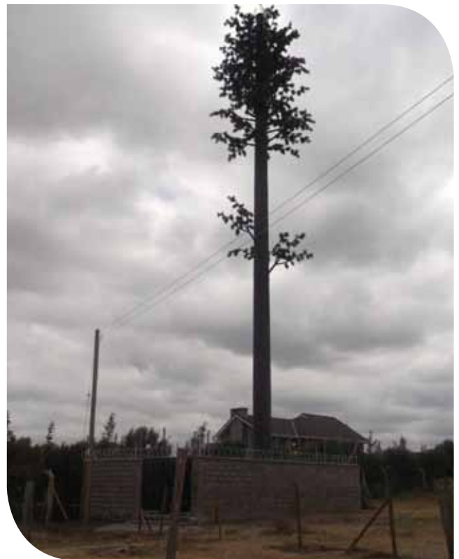
A Base Station Transceiver (BTS) site deployed as an 'artificial tree' to camouflage with the existing environment which has an aesthetic appeal as opposed to the ordinary lattice mast.
