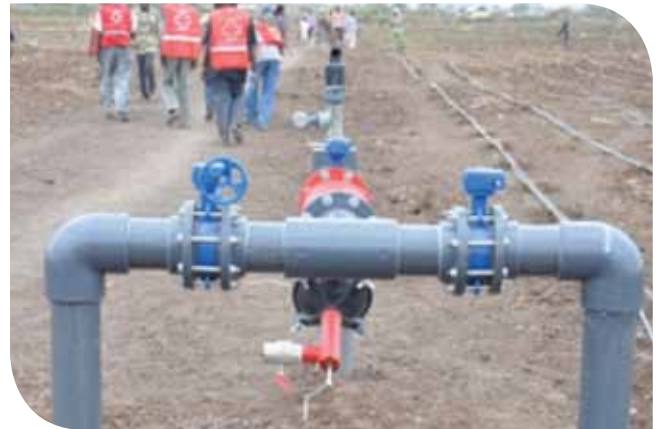
The water and irrigation infrastructure in Waldaa, Moyale on the Kenyans for Kenya farmland
